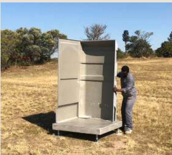
Apply a bead of Structural Polyurethane into the groove provided down the length of each side of the back wall panel
