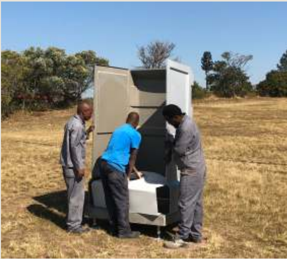
Open up the side walls slightly to fit the toilet module into place,
