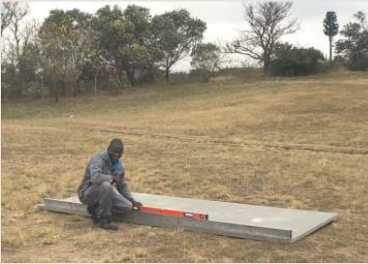
Ensure that the surface you are installing the structure onto is straight and level and set out the line of the Ablution Module you are using, ensuring that corners are 90 degrees.
