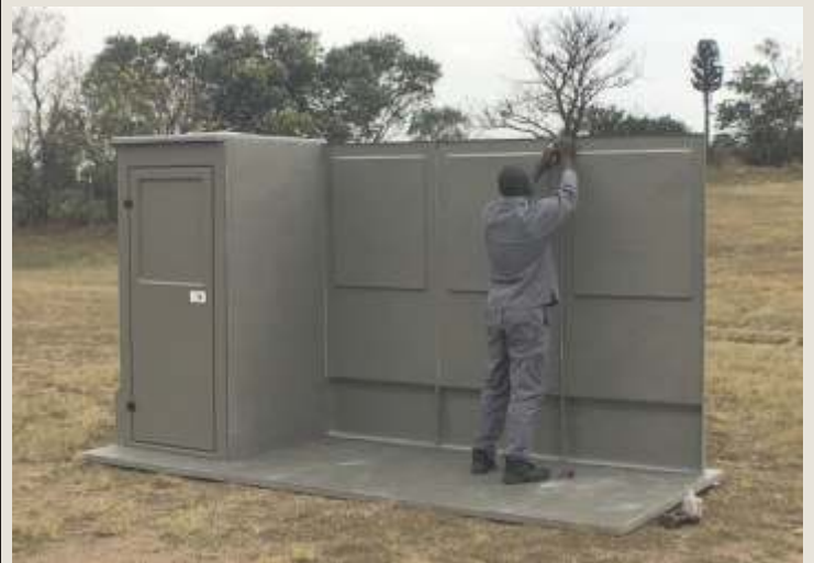
Repeat as before, attaching the next Back Wall to the previous Back Wall using 3 x M6 x 20mm machine screws provided and then fix down to the slab structure with suitable fixings.
