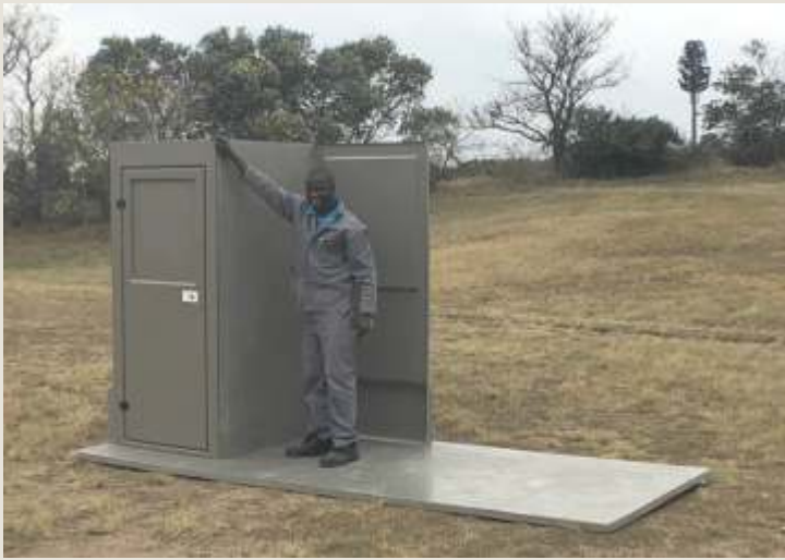
Install Mid Wall into place aligning flanges of the Back Walls and Front Door-Wall into the groove of the Mid Wall and wipe away excess Structural Polyurethane
