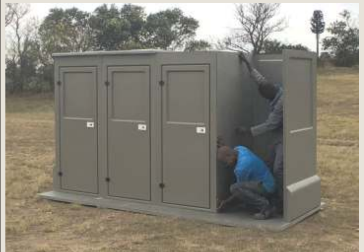
As with the previous Mid Wall, apply a full bead of Structural Polyurethane into the groove along the entire length of both sides and the top of the next Mid Wall and install into place aligning flanges of the Back Walls and Front Door-Wall into the groove of the Mid Wall wiping away excess Polyurethane
