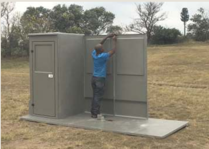
Attach the next Back Wall to the first Back Wall using 3 x M6 x 20mm machine screws provided and then fix down to the slab structure with suitable fixings.
