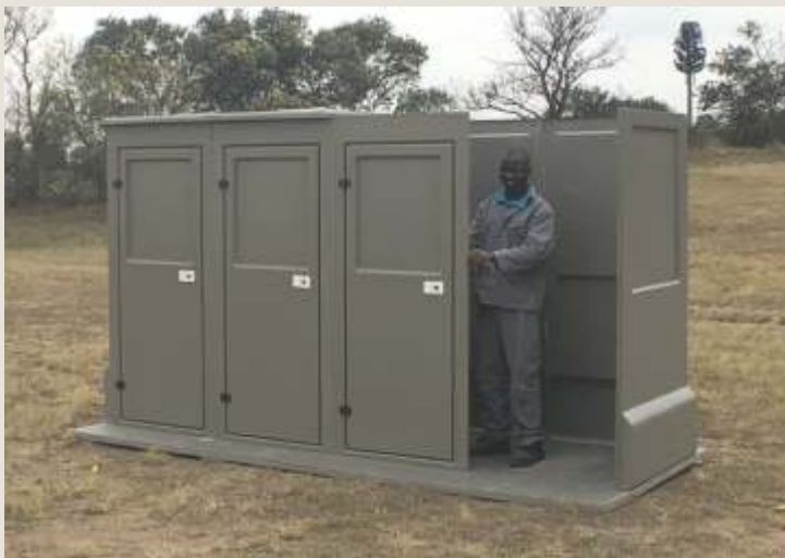
As with the previous Front Door-Wall, fix the next Front Door-Wall to the previous one, aligning the side flange of the Front Door-Wall into the groove of the Mid Wall and then fix down to the slab structure with suitable fixings.
