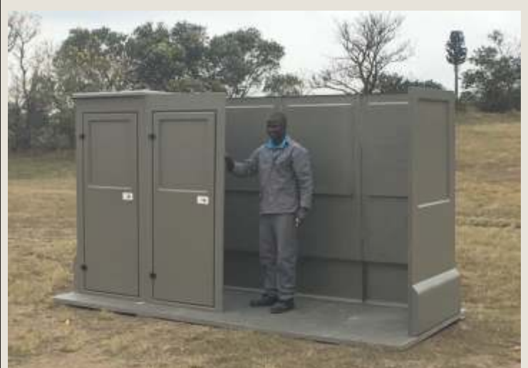
Fix the next Front Door-Wall to the last one, aligning the side flange of the Front Door-Wall into the groove of the Mid Wall and then fix down to the slab structure with suitable fixings.
